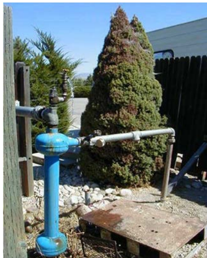
Figure 1: The wellhead on your property will typically include a pipe leading to your pressure tank.
