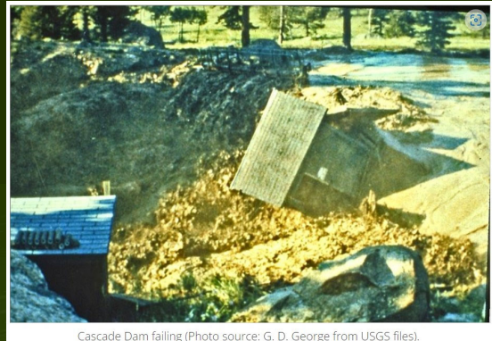
Cascade Dam failing (Photo source: G. D. George from USGS files).
